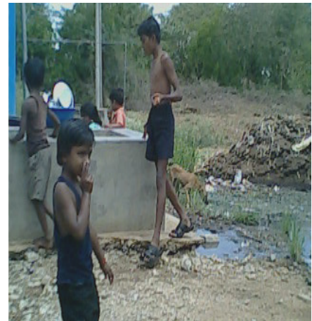
Water tank constructed GS with no drain in Kotta GP
